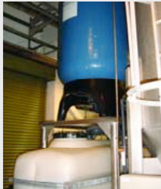
■ The raw water filtering system
