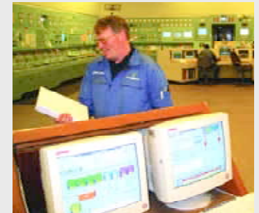
■ The station's control room
