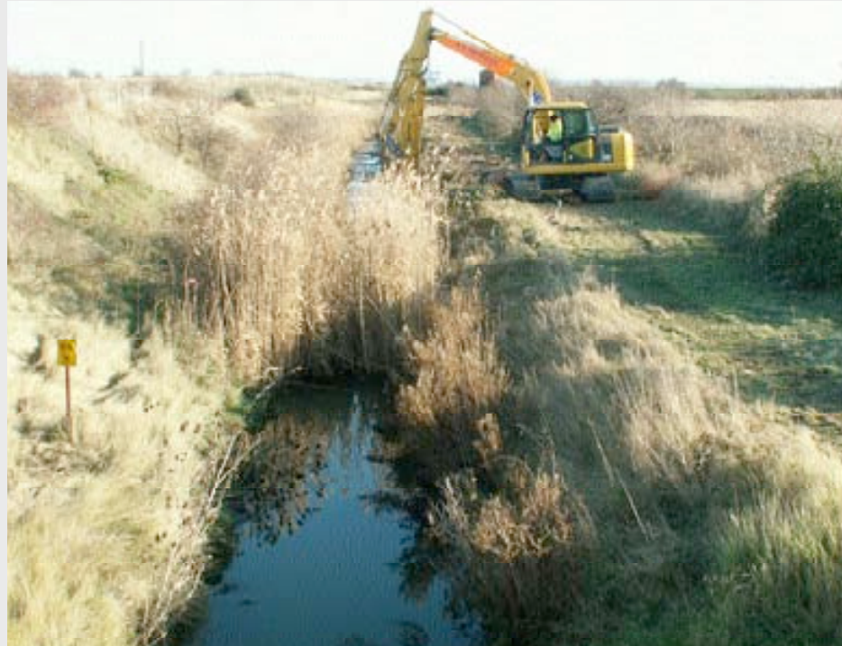
■ A digger clears out the Berry Wiggins Drain in winter 2008 to improve habitat for Water Voles
