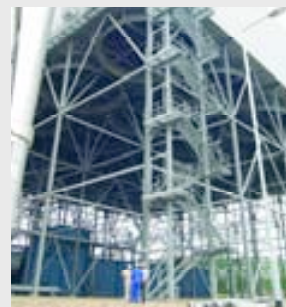
■ The air-cooled condenser
