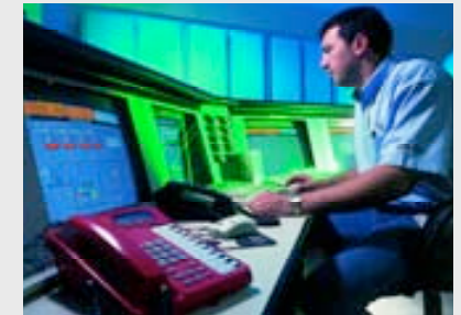
■ Damhead Creek's control room
