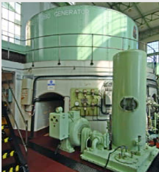
■ A turbogenerator at Glenlee Power Station
