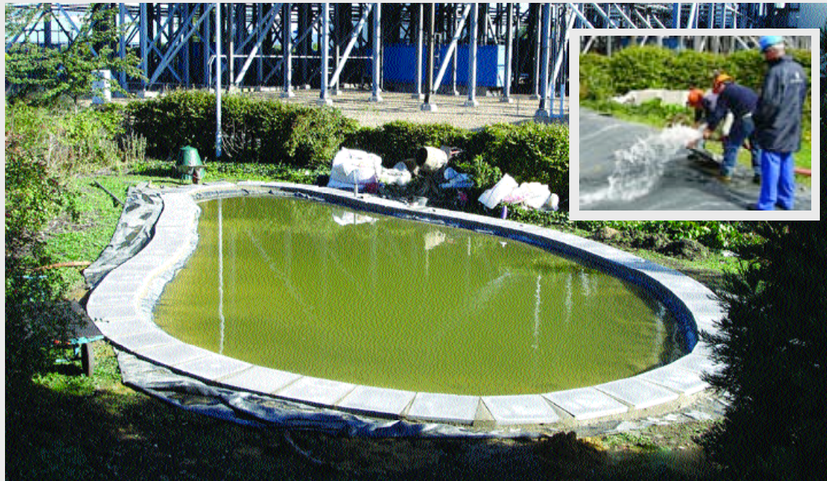
■ The pond in Rye House's wildlife garden after its construction and, inset, station staff and contractors filling it with water
