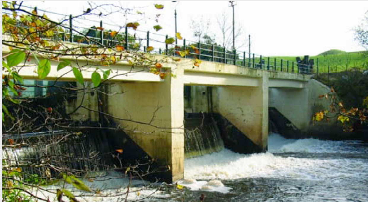
■ Bonnington Weir's bridge deck is set for major refurbishment works and (below left) recent work to install a new tilting gate
